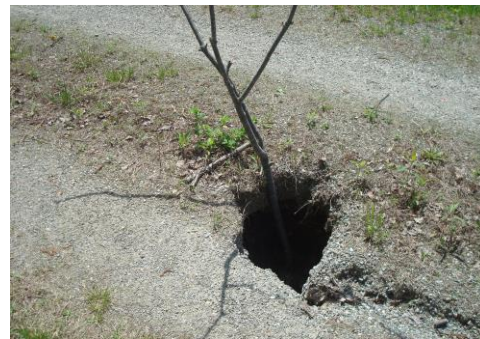
The MVRT's surface requires regular monitoring and maintenance to prevent holes like this one
