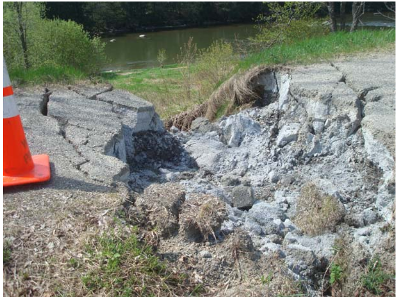
A failed culvert beneath the MVRT closed the Trail for a couple of weeks in May
